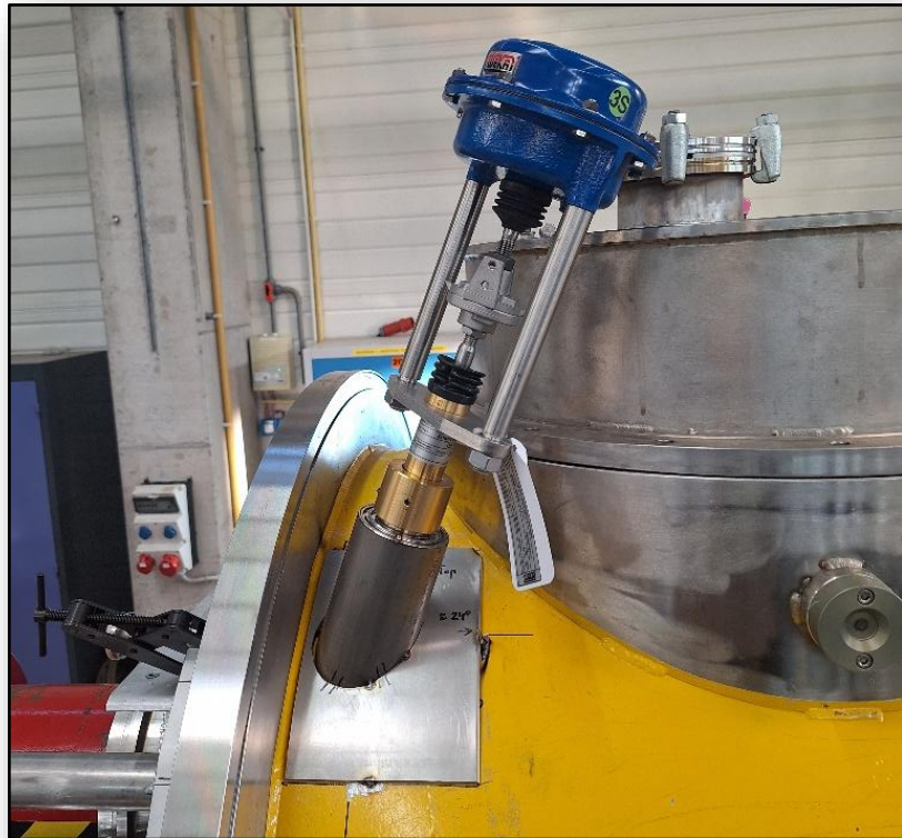
JT valve retrofitted in XM-3
